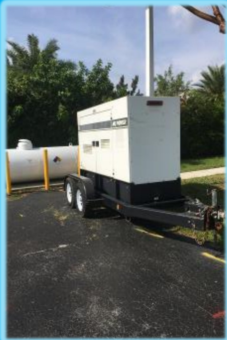
Pictured above: Temporary generator that has been deployed to ensure backup power during the transition.
